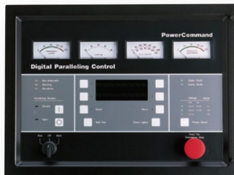
PCC3100 Premium performance and flexibility for generator sets with hydromechanical fuel control systems
